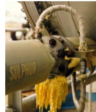
Sulfur Leakage at Flanges Without a Reduced Port Valve
